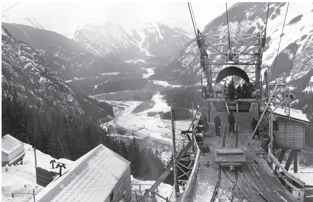
Figure 18: A penstock liner is hoisted up the mountain. It will be used to line the tunnels carrying water from the Nechako Reservoir to the Kemano powerhouse. (Tramway landing on 1600' level, 23-Jan-54. Alcan ID no. KR-1576. Alcan Collection. Courtesy of the Kitimat Museum & Archives. KMA No. 987.3.3)
